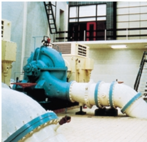
Figure 1.49 A water pumping station is needed to keep water flowing at a certain pressure through city pipelines.
